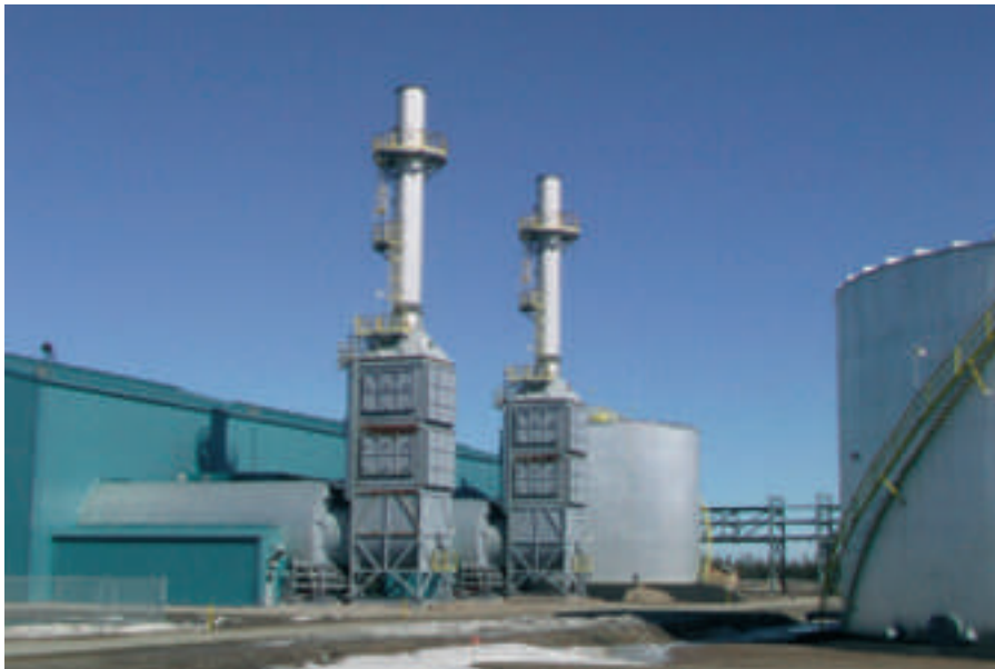
Steam generation unit at Suncor's Firebag oil sands lease, Alberta, Canada.
